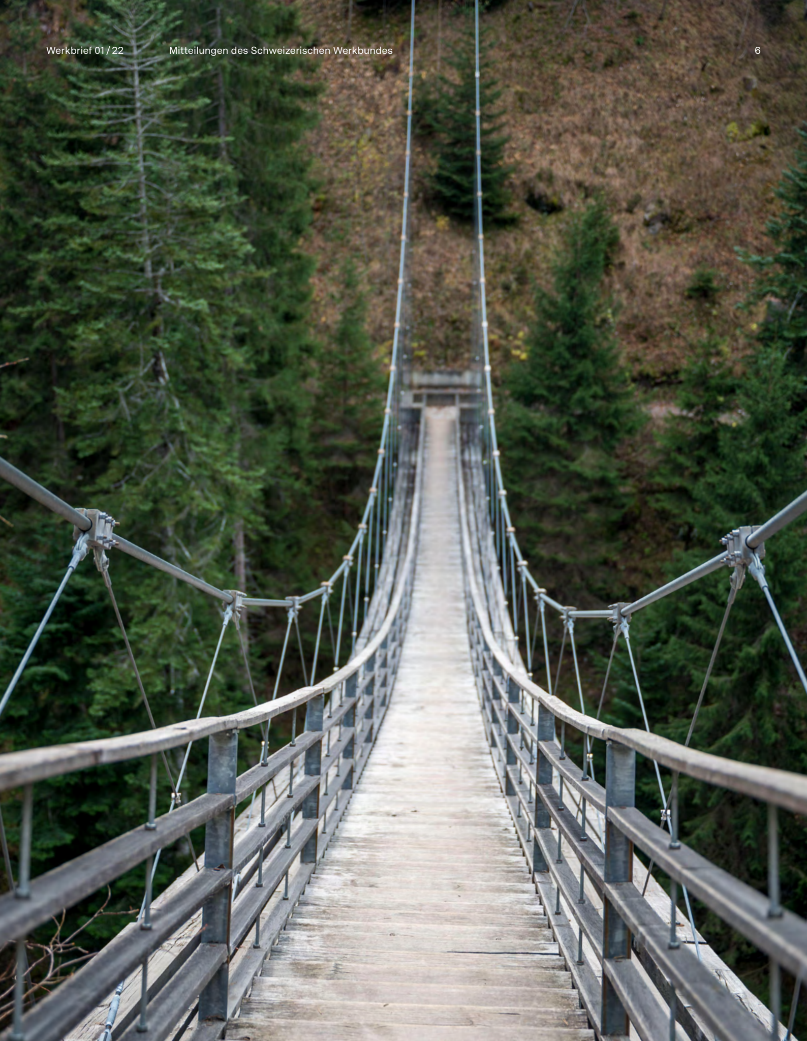
Jürg Conzetta's second Traversinersteg der Viamala as cable-stayed construction with staircase-like path. Photo: Marcel Gross.
